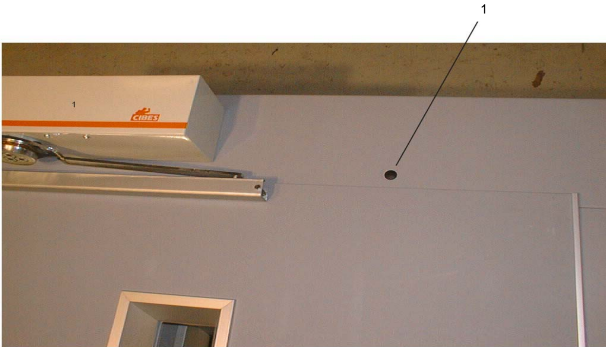
Figure 5 Emergency opening of the platform lift door from the outside
